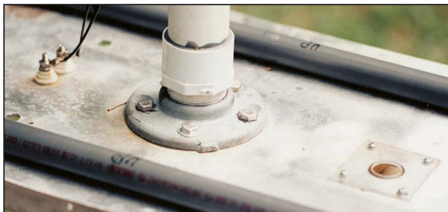
Figure 3—Galvanized pipe floor flanges are used top and bottom to connect the mast and crossover feed support. This is the top flange with a PVC adapter. The hole to the right of the flange is for a coaxial feed line for the 2-meter quad mounted above the W8JK array. Ceramic feedthrough insulators on left are for the 450 \Omega ladder line feed.
